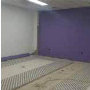
CONVERSION IN PROGRESS: left wall separates studio from main locker room and right wall completed with dry wall
